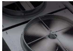
Heating and ventilation
